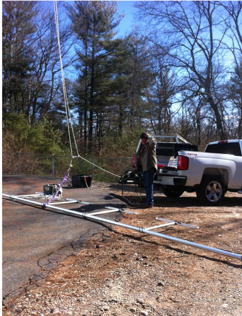
Rigging the Sinclair antenna. The new .18 repeater antenna is a Sinclair SD214-SF2P2SNM(D00) 4 dipole, 8.0 dBd, bi-directional, N-Male, 138-174 MH
