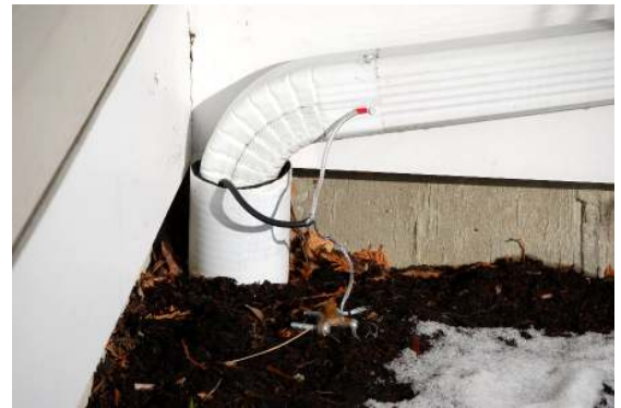
Attachment to gutter downspout and shield to ground rod
