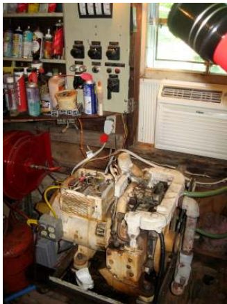
Motor – Generator and barn heater
