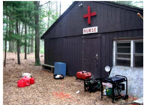
Emergency generators at main pavilion
